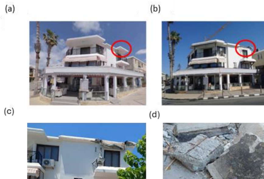
Figure 1: (a) Building facade (the failed cantilever is discernible) (Durable Structural Consulting Engineering Archive); (b) Building facade (the failed cantilever is visible) Durable Structural Consulting Engineering Archive); (c) and (d) Photographic documentation of the failure of the 165 cm cantilever (Durable Structural Consulting Engineering Archive).
