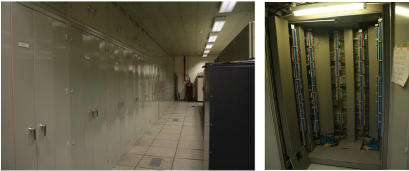
Fig. 1. I/O Cabinets and wiring cabinet.
