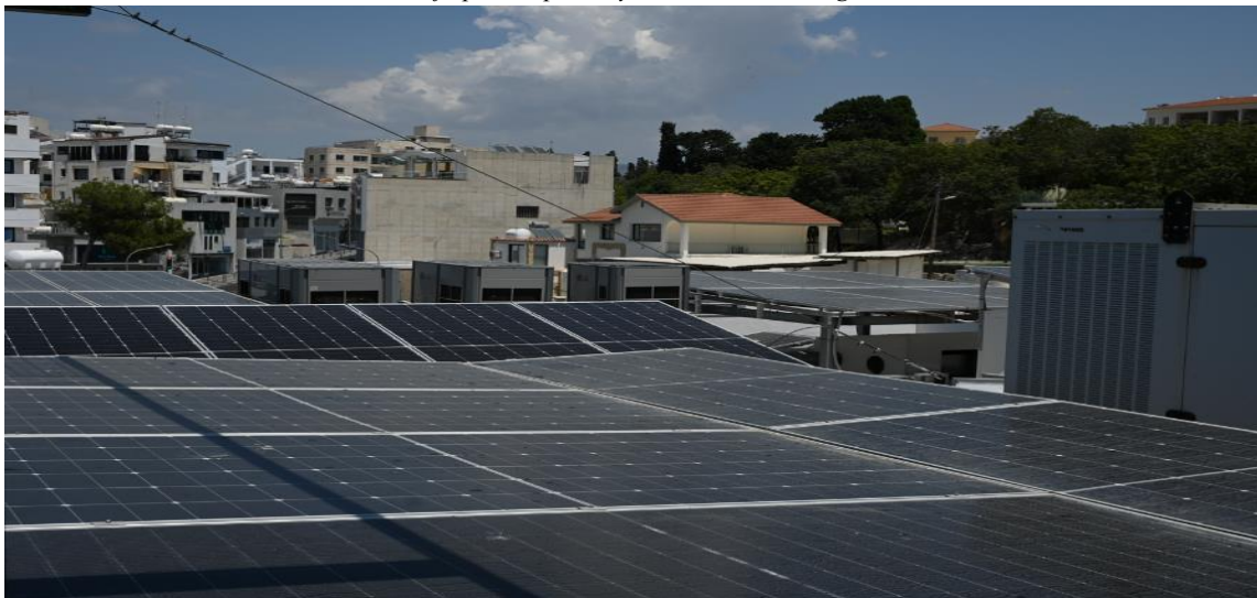
Figure 2. Rooftop solar panels at Be.On Paphos Source: Author's photograph, 2026.
