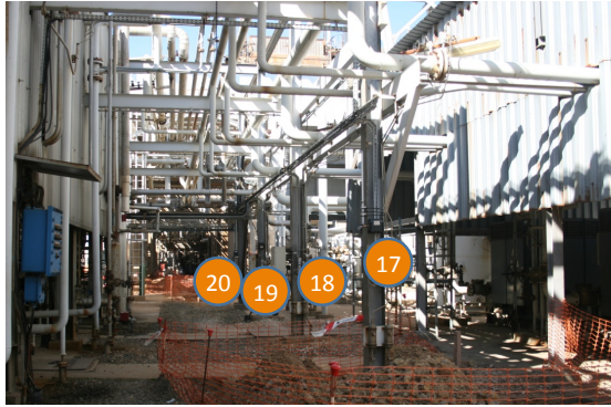
Figure 3. Sines testbed photo showing nodes 17 to 20 (front to back)
